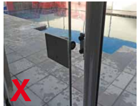
The gate or components may need to be adjusted or replaced to ensure self-closing mechanism works properly.
